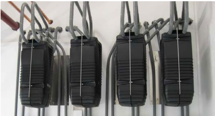
Vulcans installed back to back.
